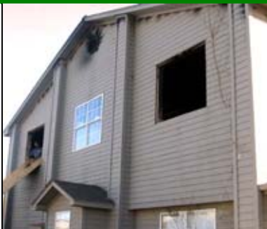
Building burned in the fire
